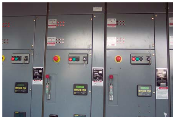
Power control room
